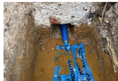
Pipe entering property through duct
